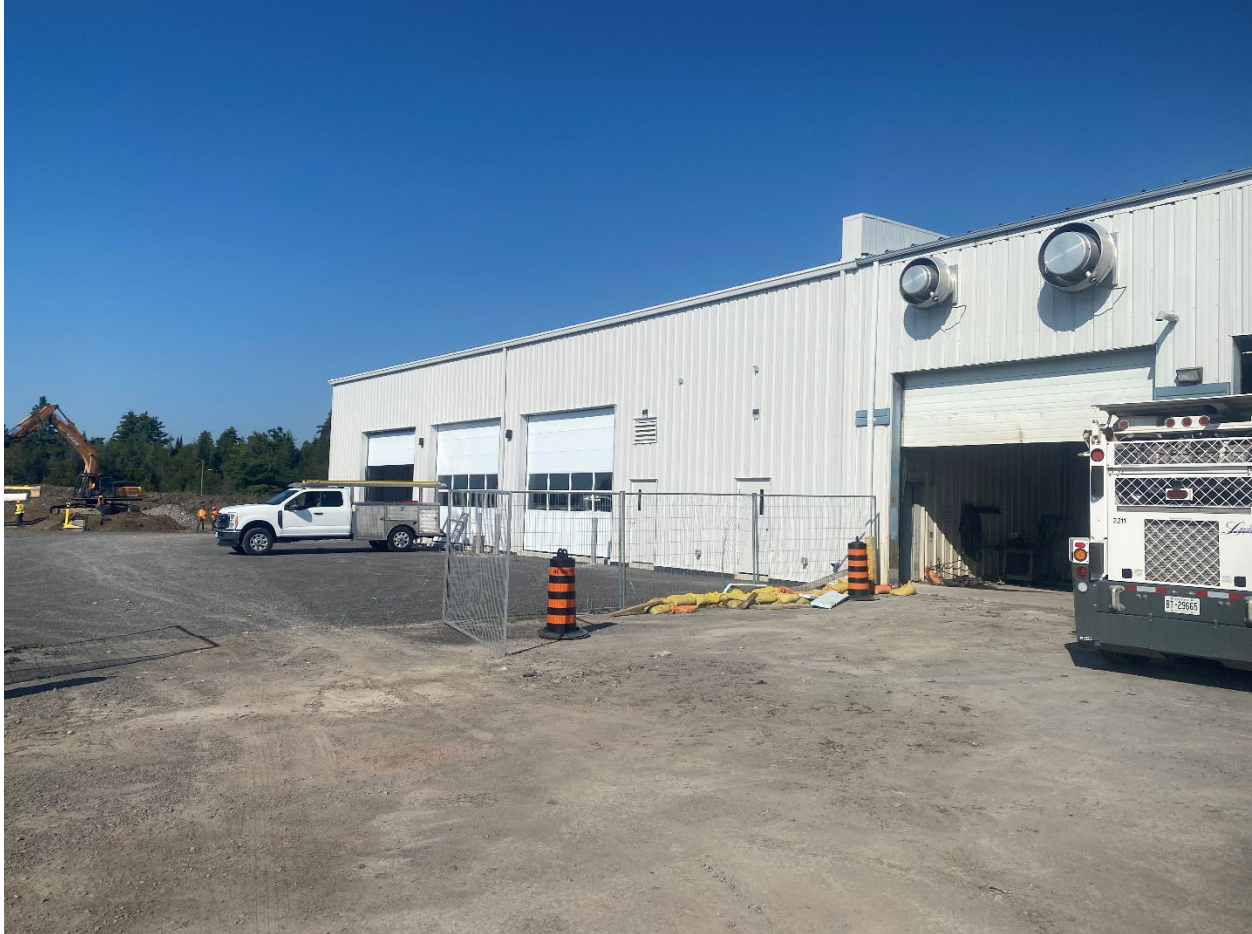
Figure 2 Exterior of Public Works Garage, showing original rear wall and expansion area
